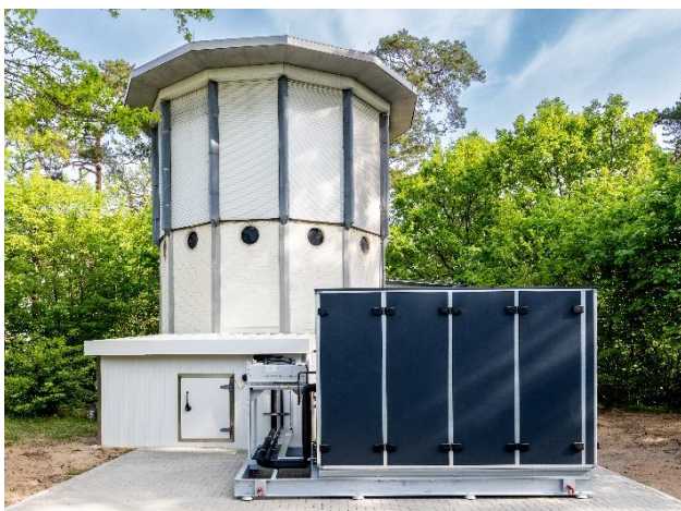
Figure 1 DLR's rotor tower with the cooling system
