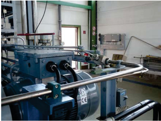
Figure 5: Upgrade of compressor motors
